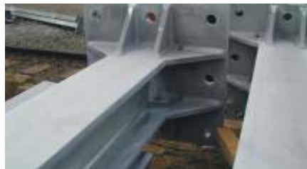
Concealed cracks after MT-testing in the area of a stiff pedestal of a post
