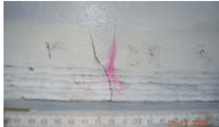
Concealed galvanizing crack (MT tested) adjacent to a wide open crack (PT tested) in the frame of a girder with welded bracket as well as indications of longitudinal cracks in the weld metal
